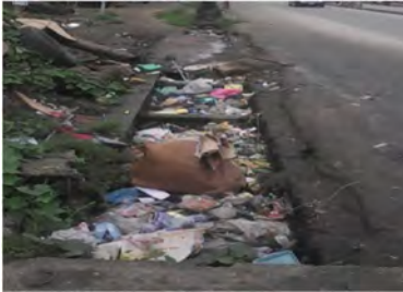
Plate 7: Blockage of drainage with Wastes
